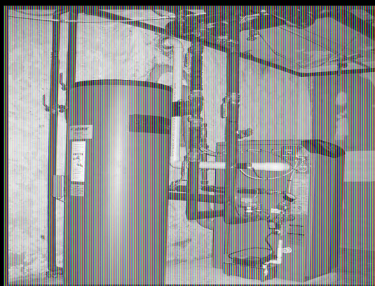
Boiler With Storage Tank
